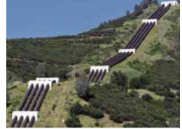
Water Supply & Transmission Pipeline
